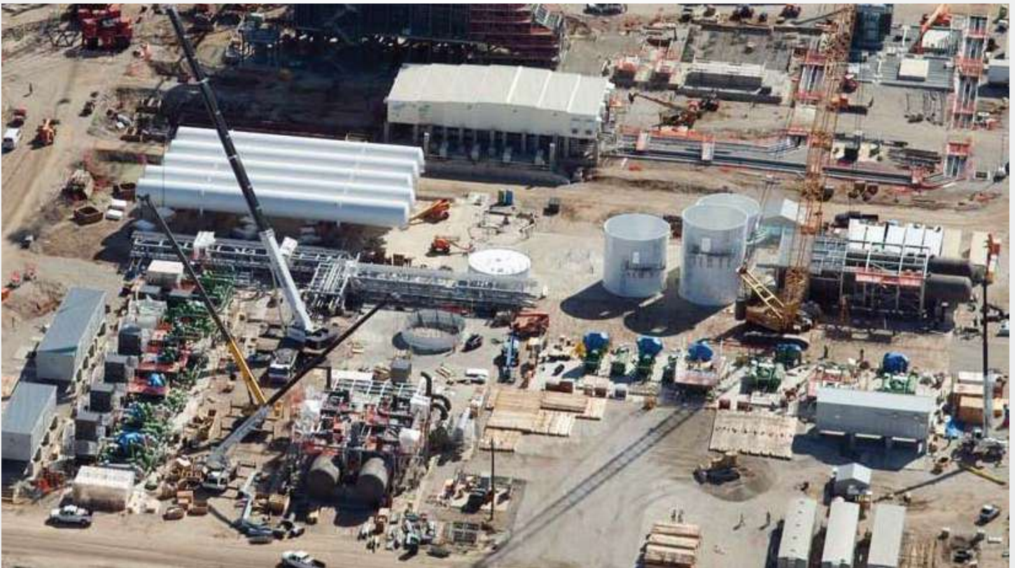
Work site for construction of an IGCC power plant in the US. Ingersoll Rand field service technicians were on site to coordinate the installation and commissioning of thirteen MSG-16 compressors.
